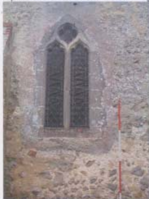
▲ Fig 17: Eastern-most window in the south wall of the nave, inserted in the 1850s, with evidence of a series of repairs to the masonry to correct subsidence.
