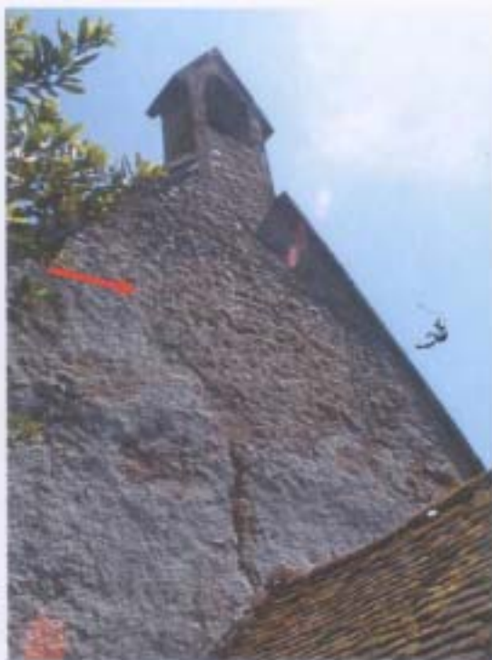
► Fig. 16: West wall of Chithurst church showing scar of removed rose window and settlement cracks above the roof line of the porch, worsened by the downward thrust of the bell cote above. (Robert Hutchinson)
