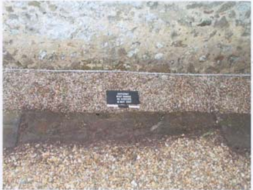
► Fig.40: Worn and badly cracked floriated cross slab, (Slab 2), fourteenth-century, probably to a priest; second from the east in the line of slabs running east-west in path alongside north wall of Chithurst church.
